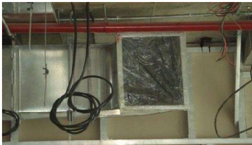
Ducts Wrapped With Plastic To Avoid Dust Plastic
